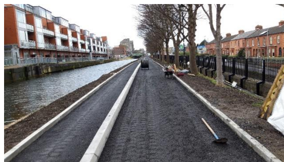
Kerbing installed on north side towpath between Cross Guns Bridge and Lock 4
