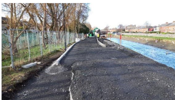
Kerbing installation on south side of canal between Binns Bridge and Lock 3
